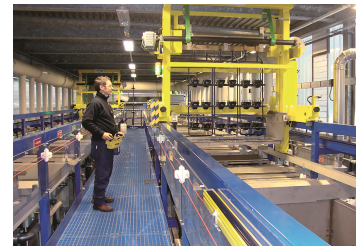
ECP surface treatment plant
